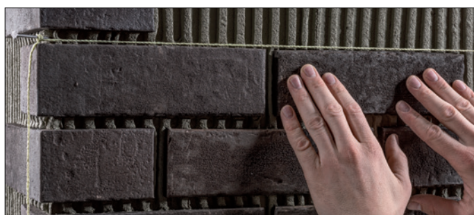
Placement of the surface clinker brick slips using a line aid. The clinker brick slips are pressed into the adhesive bed.
